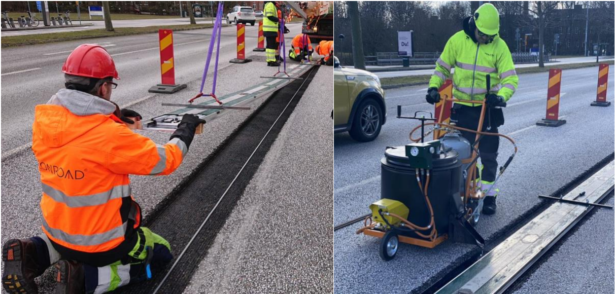
Figure 3-2 Left: Installing the ERS, Right: Moulding the ERS into the groove in the road.
