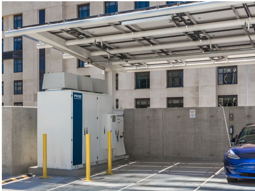
Figure3: Modular 250kW/650kWh Microgrid System in Single Parking Stall Under a PV Canopy
